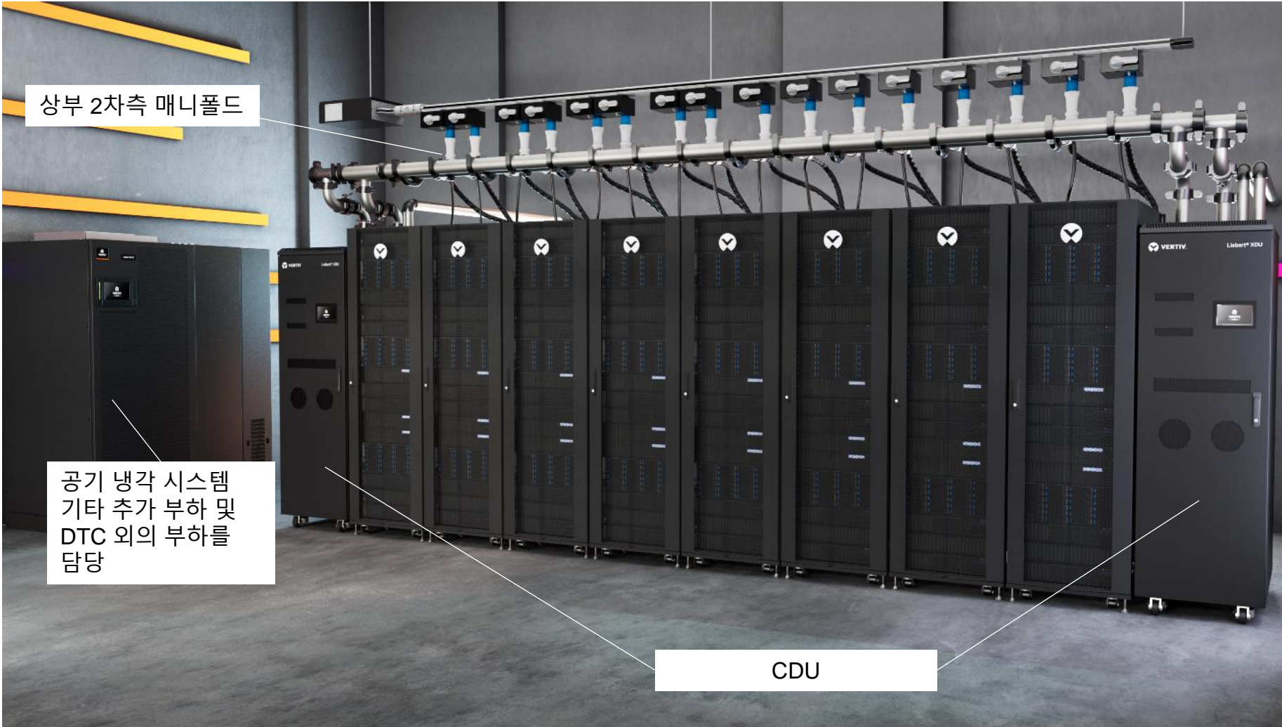
Liquid Cooled Row of IT with Redundant Cooling Distribution Units (CDU's)
